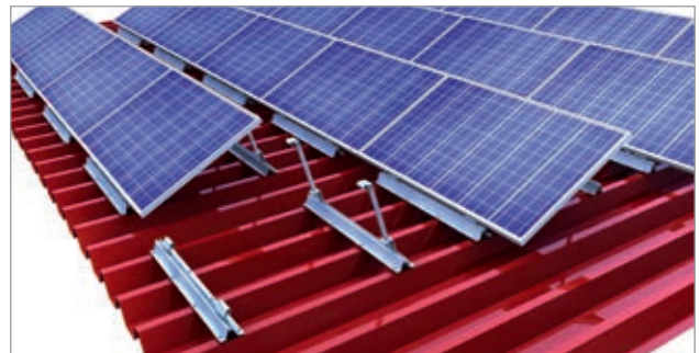
Clamping system: South-facing
